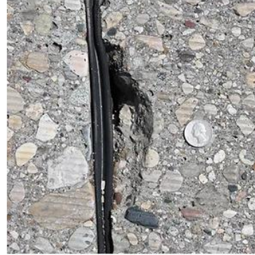
Spalled Joints and Cracks
