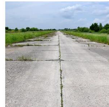
Joint Sealant Failure
