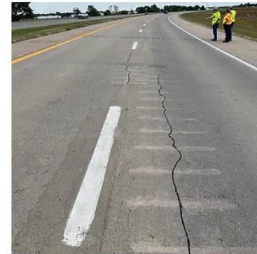
Low-Severity Longitudinal Cracks or Joints
